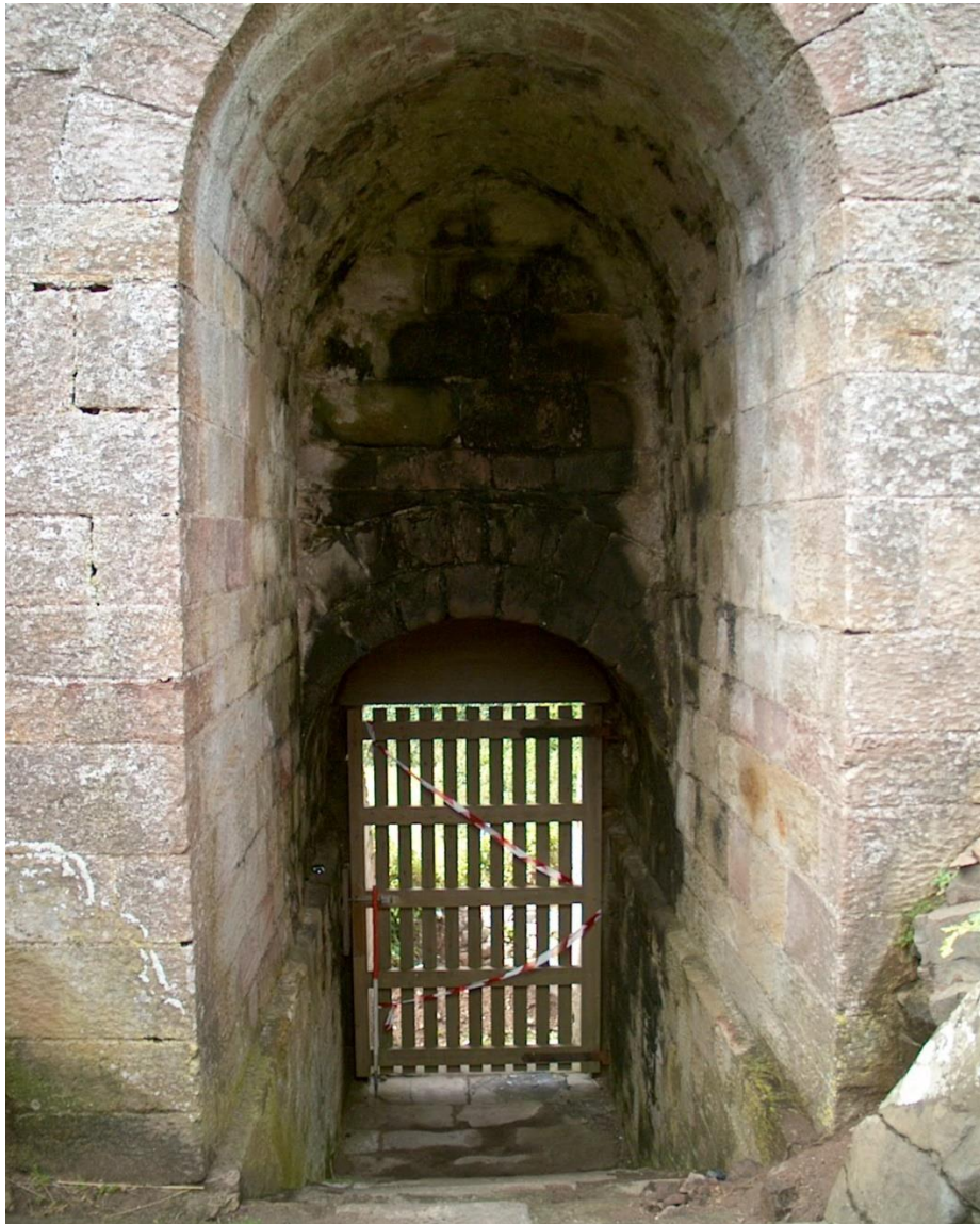
Figure 7: Interior of the curtain wall showing the vaulted passage and the interior of the gate arch, facing south-west
