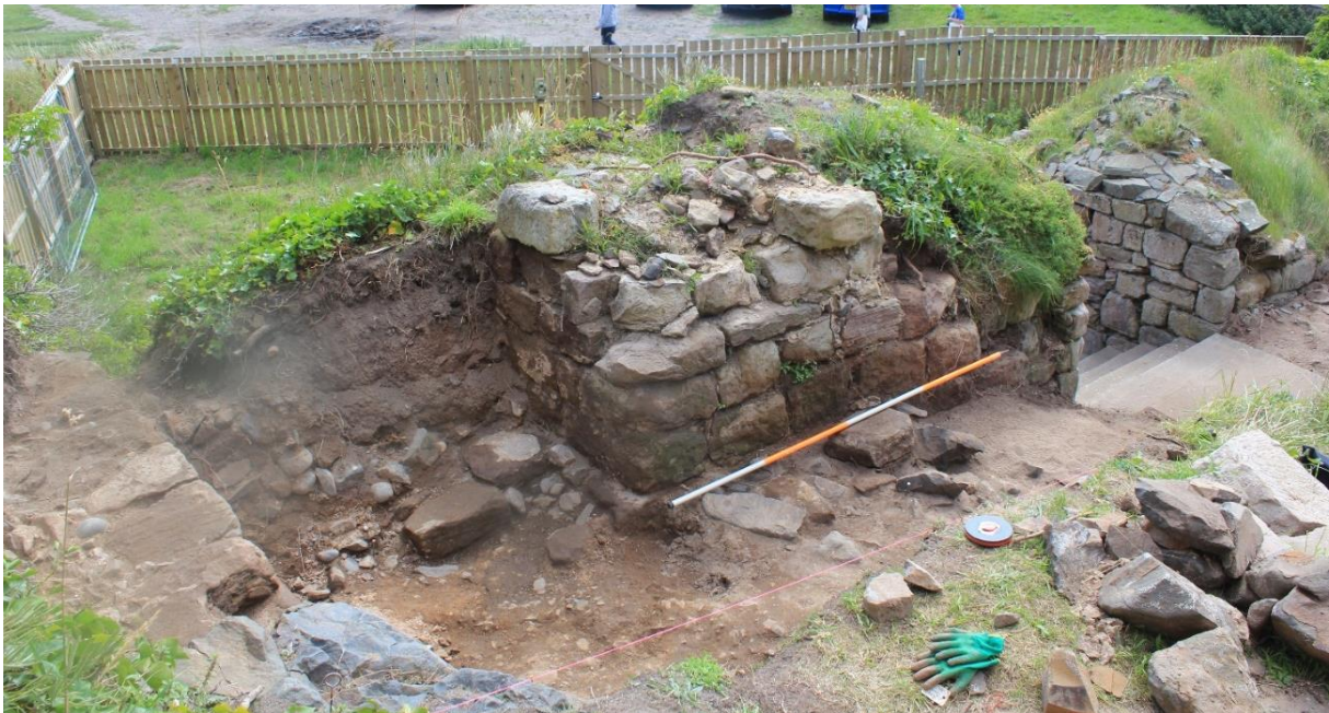
Figure 13: The recently discovered blocked doorway in wall W1 (see Figure 2 ) with some of the blocking still in place, facing south-west
