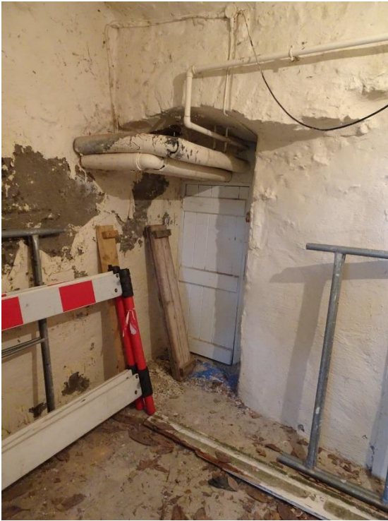
Fig. 42: Interior of south gate-tower room G5, looking northwest showing passage doorway G2b-3
