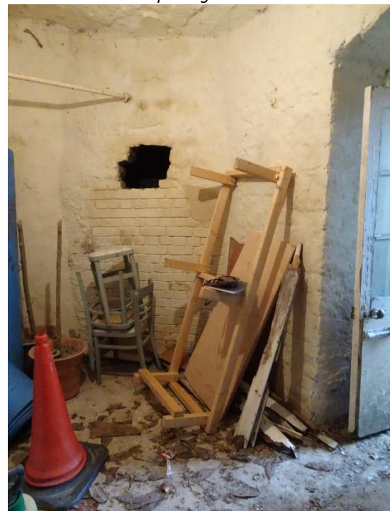
Fig. 45: Interior of south gate-tower room G5, looking southeast showing possible blocked opening G5-2
