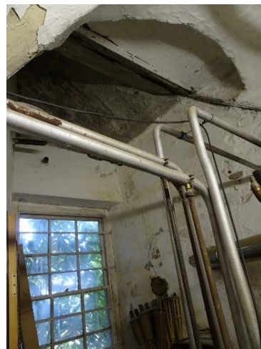
Fig. 75: Southern undercroft eastern bay G10a looking southwest, up into the head of altered embrasure G10a-3
