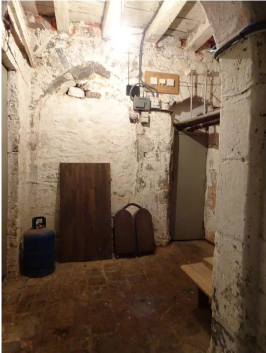
Fig. 36: Medieval doorways G2b-1 and G2b-2 on the north side of the passage, looking north
