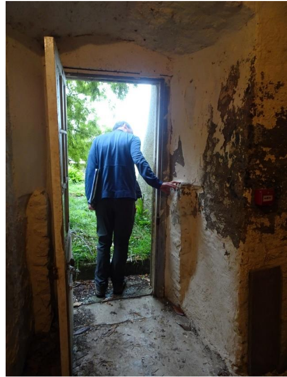
Fig. 43: Interior of south gate-tower room G5, looking southwest showing external entry G5-3, enlarged from a medieval loop or light
