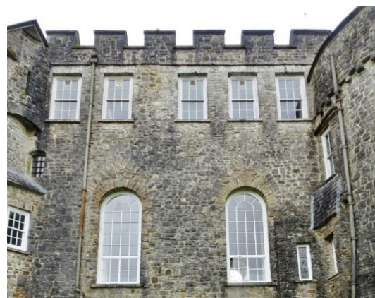
Fig. 173: North wall of central block, looking south, showing blocked chutes/sockets (beneath upper floor windows)
