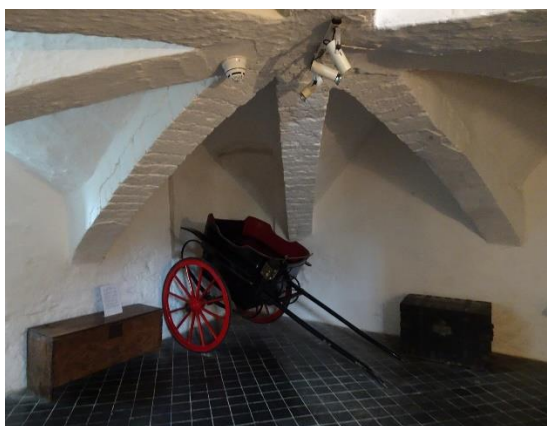
Fig. 50: Northeast Tower room G6, looking southeast, showing blocked gate-passage doorway G2b-2 (behind carriage)
