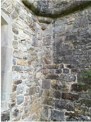
Fig. 80: Northeast face of the Northwest Tower, showing evidence of blocked entry G11a-1
