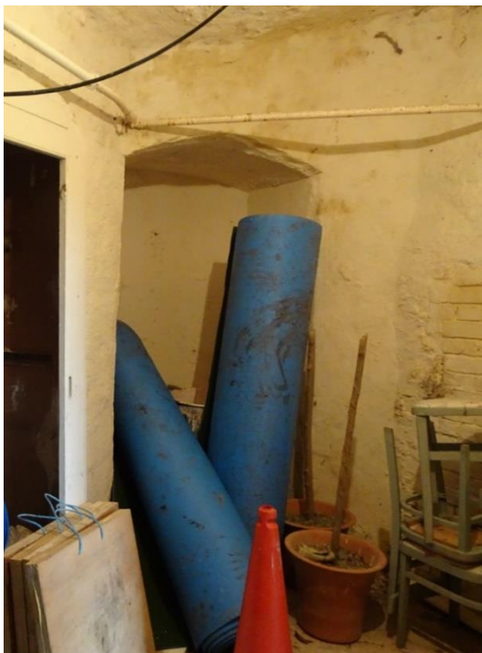
Fig. 44: Interior of south gate-tower room G5, looking northeast showing blocked opening G5-1
