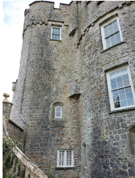
Fig. 41: Exterior of north gate-tower, looking south, showing ground-floor window G4-1, first-floor light F13-2, blocked second-floor light S22-2 and third-floor window T31-4
