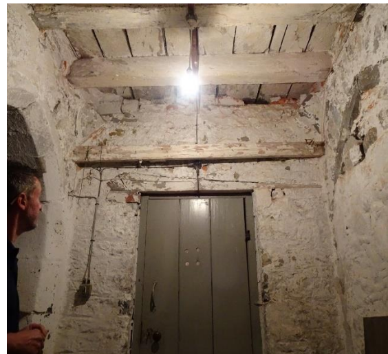
Fig. 39: Springers for medieval arch G2b-5, now infilled by post-medieval walling, looking west
