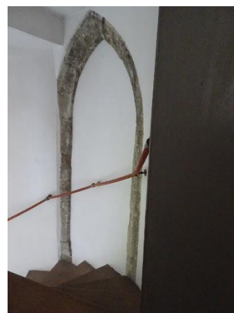
Fig. 136: Blocked medieval doorway S25-5 between spiral stair SSB and room S25, looking northeast from stair
