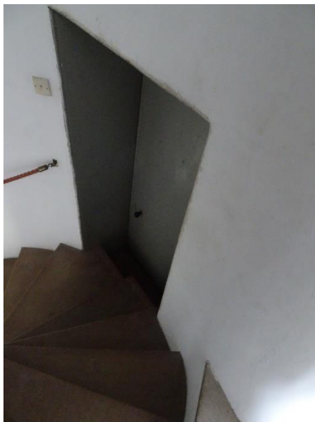
Fig. 149: Doorway S28-1 between spiral stair SSB and the Great Hall gallery, looking southeast from the stair
