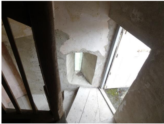
Fig. 166: Spiral stair SSB caphouse, looking west at: (L-R) recess of former entry onto Great Hall north parapet; slit-light SSB-4; modern entry onto Northeast Tower parapet
