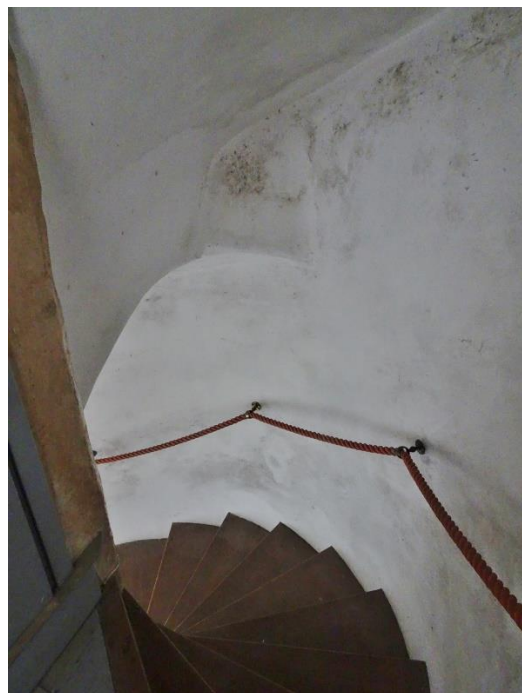
Fig. 165: Looking down at spiral stair SSB from inserted doorway T33-1, showing vaulted roof
