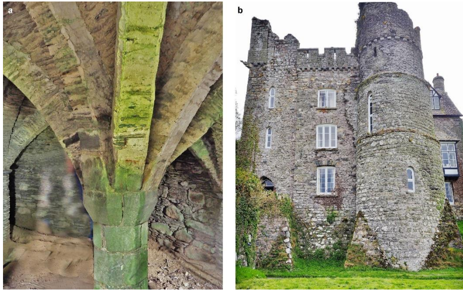
Fig. 197: Newport Castle (Pemb.), c.1300-10: a) rib-vaulted undercroft; nb. pier apparently rebuilt; b) external view of gatehouse (photos Neil Guy)
