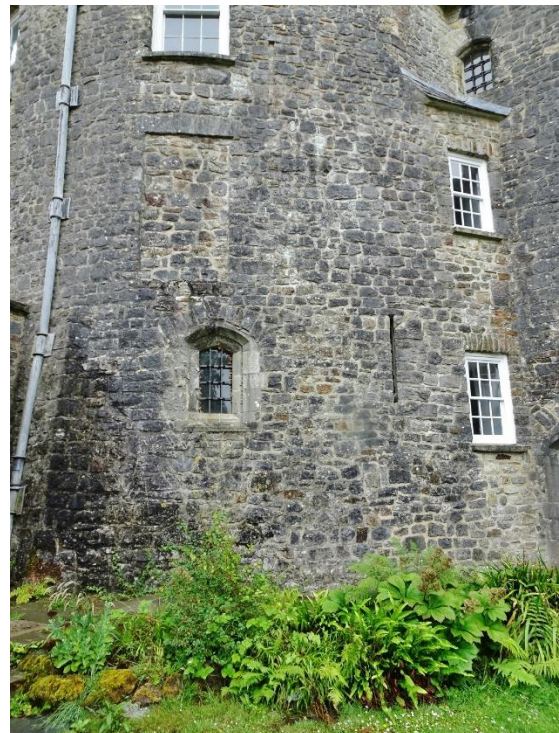
Fig. 61: The Northeast Tower from the northwest, showing openings (some blocked) including spiral stair window SSA1, with modern surround (left of centre), and two windows plus a slit-light in stair SSB (to the right).
