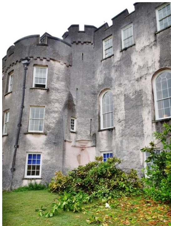
Fig. 110: External view of corbelling between the Southwest Tower and the Great Hall, carrying passage F20 and spiral stair SSC, looking northwest
