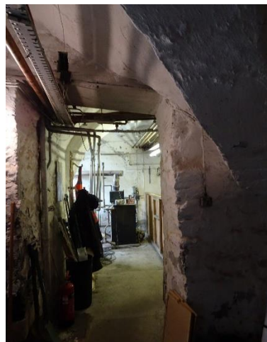
Fig. 59: Southeast Tower room G7a, looking west, showing post-medieval entry G7a-2 into the central undercroft
