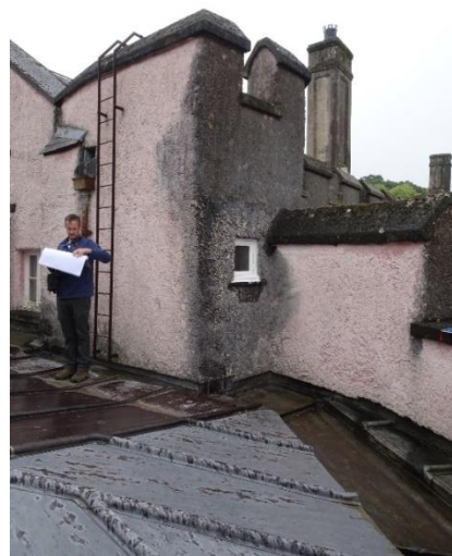
Fig. 169: Spiral stair SSC caphouse, external view looking northeast from Southwest Tower parapet
