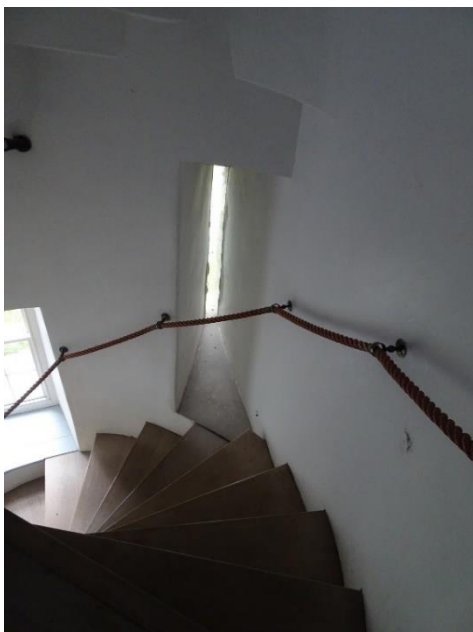
Fig. 62: Spiral stair SSB – internal view of slit-light SSB-1, between ground- and first-floor levels
