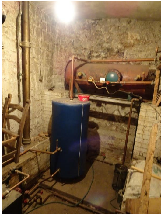
Fig. 40: Interior of north gate-tower room G4, looking northeast, with modern boiler apparatus
