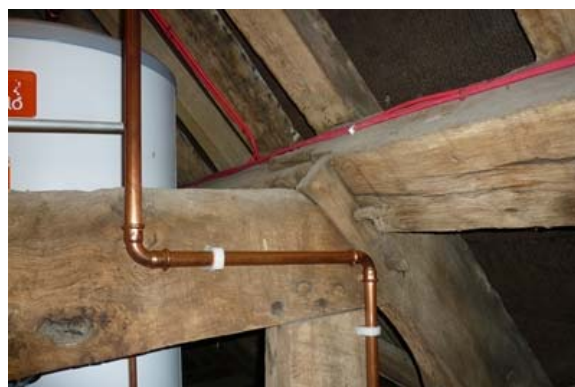
Photo 14: North range – diminished principal rafter
