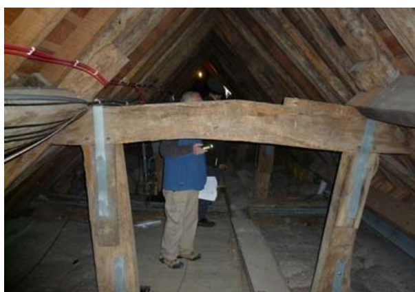
Photo 19: East range – truss 11 with diminished principal rafters
